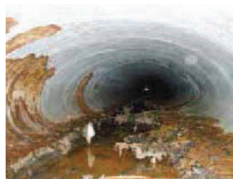
Damaged corrugated metal culvert.
