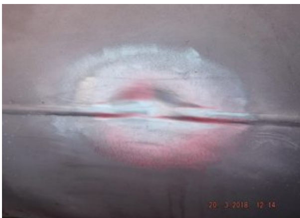
A carbon steel crude oil pipeline had sustained a dent and a related crack in a seam weld.
