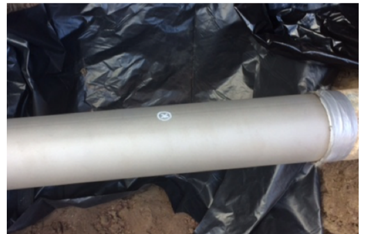
Defect within seam weld.
