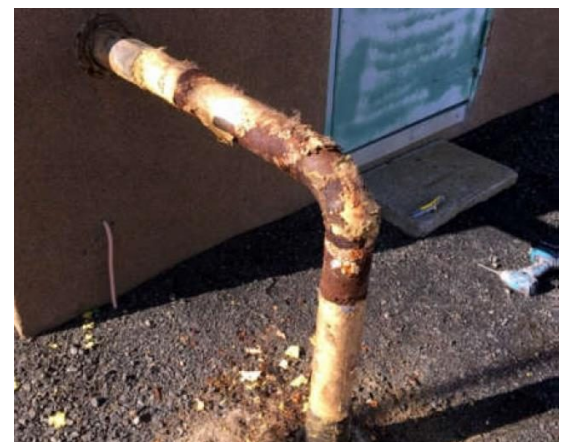
Defect after removal of insulation
