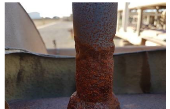
Area of external metal loss
