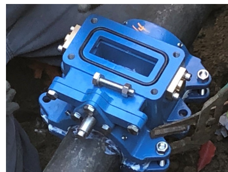
Valve body installed on pipe
