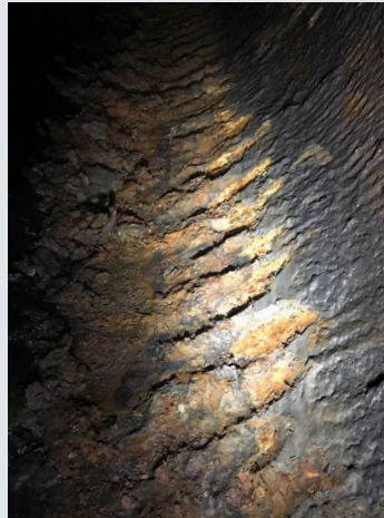
Before: Sewer showing signs of deterioration of existing concrete and heavy scale and sediment build up.
