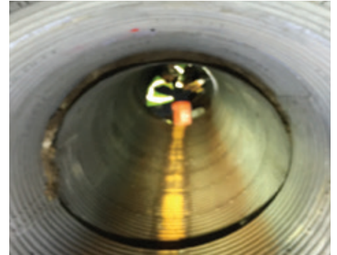
Example of joint separation in CMP culvert.
