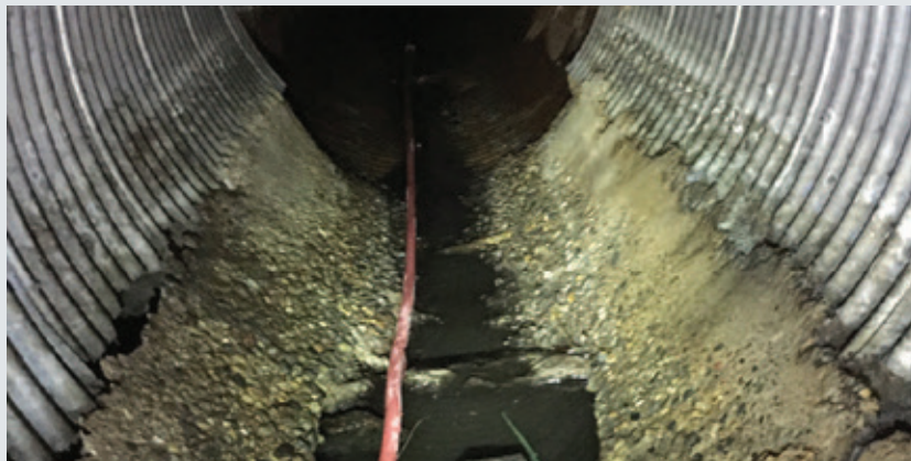
Damaged paved invert from previous repair.
