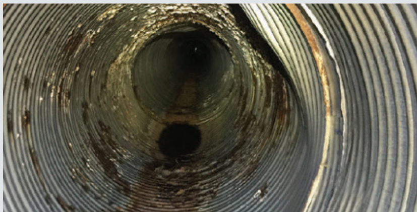
Example of corrosion near joints.
