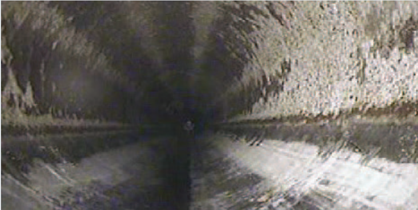
CCTV footage of RCP pipe prior to repair, showing corrosion.
