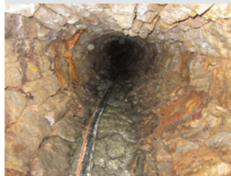
Corroded stacked stone sanitary sewer.
