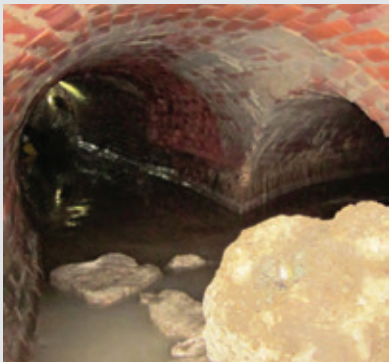
Pipeline diverging and changing sizes.
