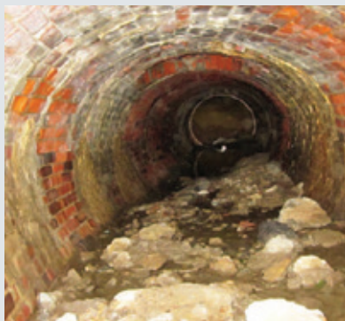
Large debris inside circular brick pipes.
