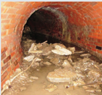
Significant curvature of existing structure.
