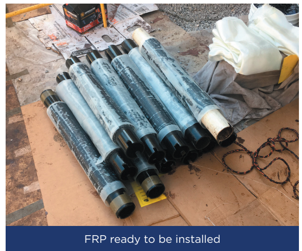
Unit 3 cooling water pipe
