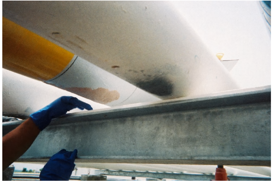
Corrosion at pipe supports
