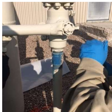
Pipe supports are installed to limit the effects of corrosion and the environment for the gas transmission lines.
