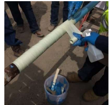
CSNRI trained and certified technician apply Contour WA™ to a prepared line.
