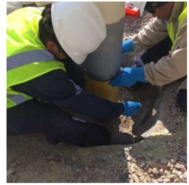
Installers secure Snap Wrap to strengthen the pipe and protect it at the air/soil interface.
