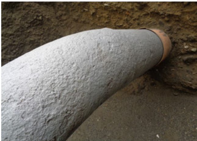
Figure 1. Transmission pipeline suffering from general external corrosion.
