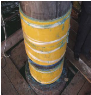
The completed repair with Clock Spring sleeves installed both below and on top of the welded steel sleeve (photo: ClockSpring | NRI)
