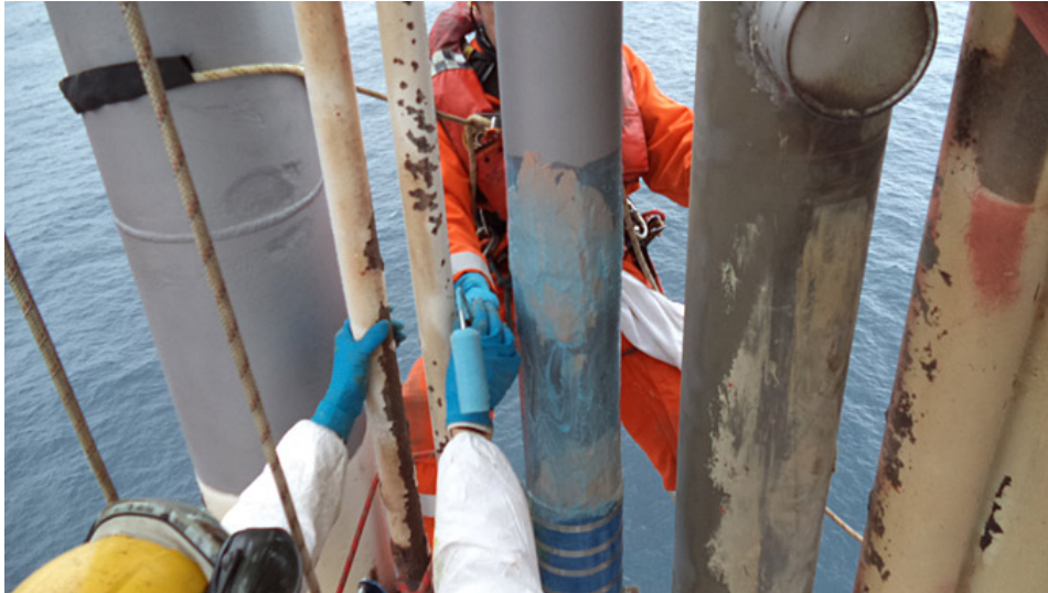
Using rollers to apply adhesive, the installation team places and secures composite sleeves on the riser (photo: ClockSpring|NRI)
