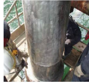
The riser is cleaned to remove all surface contaminants, revealing clean, white metal per NACE 3 surface preparation and is ready for the installation of the Clock Spring repair sleeve (photo: ClockSpring | NRI)
