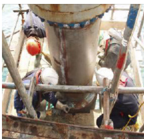
Technicians prepare the surface of the riser using 7-inch (17.8-cm) grinding machines fitted with wire wheels for larger surface areas and 4-inch (10.2 cm) grinding machines for the weld area (photo: ClockSpring|NRI)
