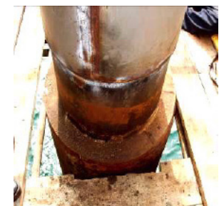
Damage was sustained on a section of pipe that had been welded, producing a surface that was not aligned (photo: ClockSpring|NRI)
