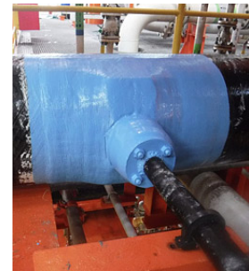
With the Thermo-Wrap™ Inspectable ECR installed on the joint between the 508-mm (20-inch) and 51-mm (2-inch) GRE lines, technicians covered the repair with 2 layers of UV-stable epoxy to protect the repair from future corrosion and abrasion
