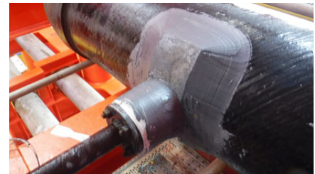
Technicians used a proprietary composite injection system to arrest the live leaks and Syntho-Poxy™ 101 to improve the complex geometry of the lines
