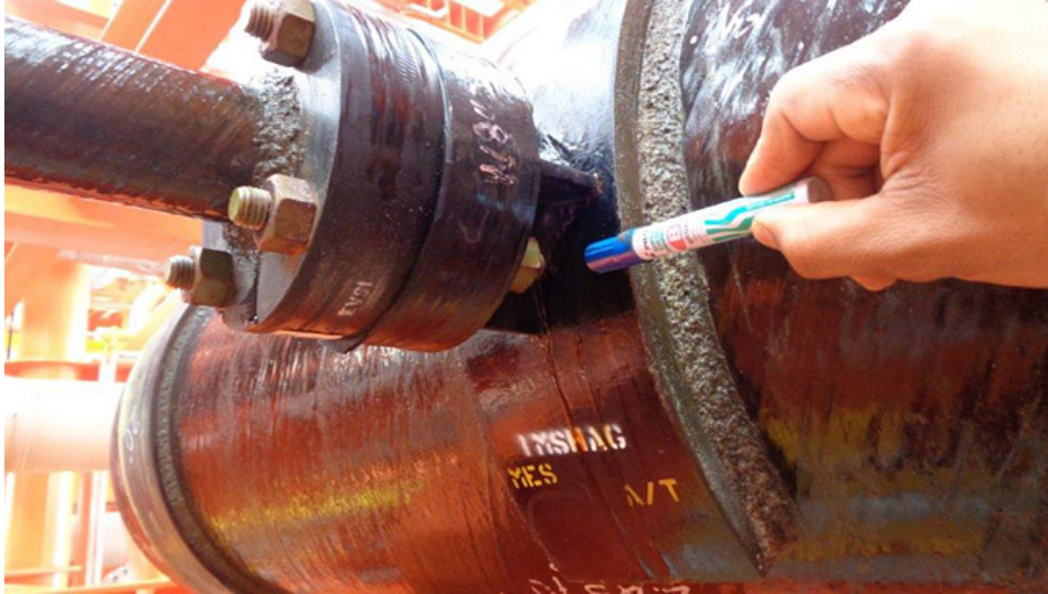
A leak is detected on a joint between a 508-mm (20-inch) and 51-mm (2-inch) GRE branch line (photos courtesy of ClockSpring | NRI)
