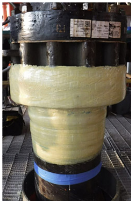
With the leak sealed, technicians applied 8 layers of the Thermo-Wrap™ Inspectable ECR to the 355-mm (14-inch) line
