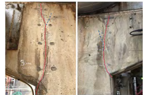
Severe cracking to concrete plinth
