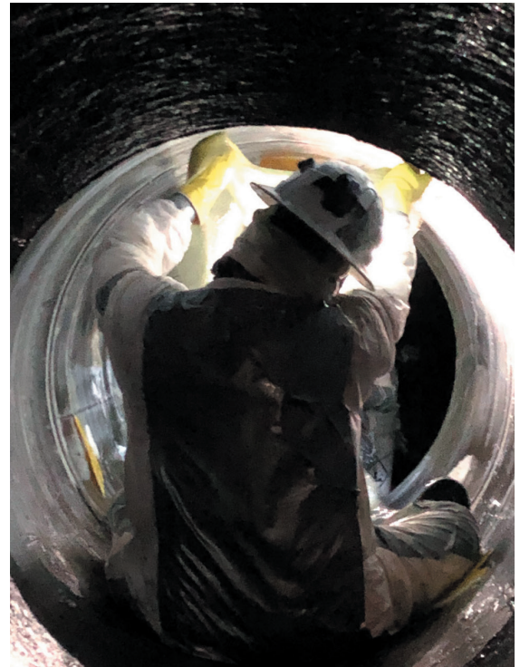
Lake Houston pump station intake piping
