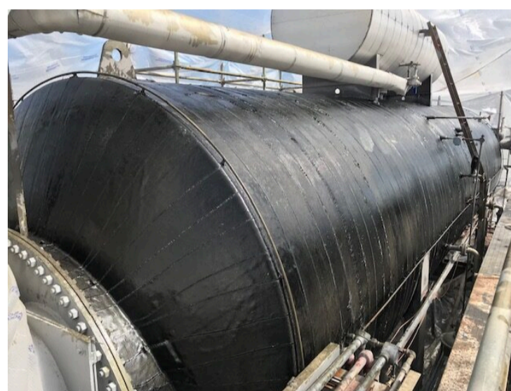
The flexibility and low profile of the DiamondWrap composite system allow installation even in areas with limited clearance. (Photo courtesy of CSNRI)
