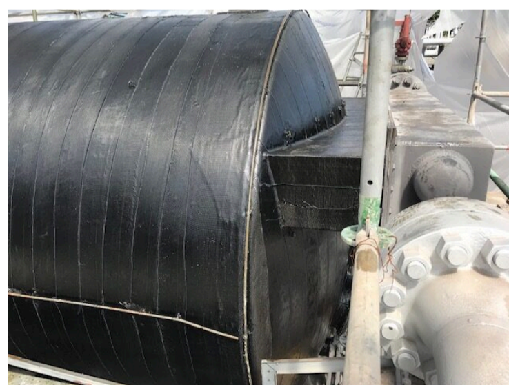
DiamondWrap can be installed on tees, elbows, and varied geometry without compromising the integrity of the repair. (Photo courtesy of CSNRI)
