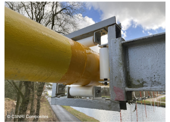
Once the system fully cured the retaining clips were removed and the existing coating extended over any surface preparation. New Pipe Support contact point rollers were also installed.
