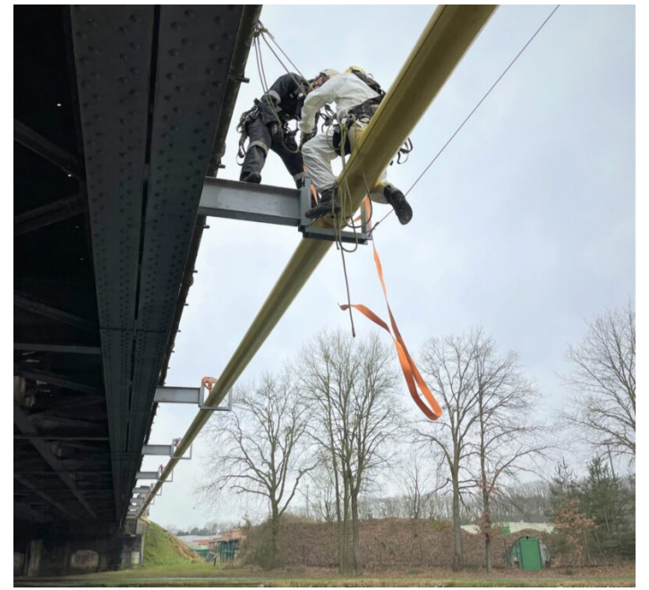
The repair area was accessed through a system of ropes and harnesses that lowered the crew to the pipe location.
