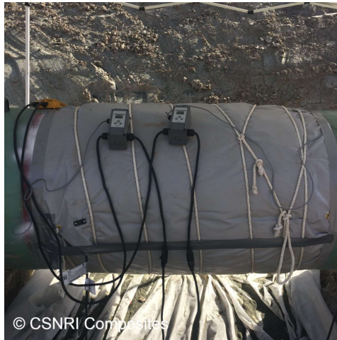
A heat blanket was applied over the constrictor wrap to expedite the curing process.
