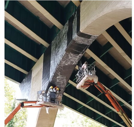
Installation of “L” Wraps of Fyfe’s Tyfo SCH-41 2X CFRP System for Shear Reinforcement
