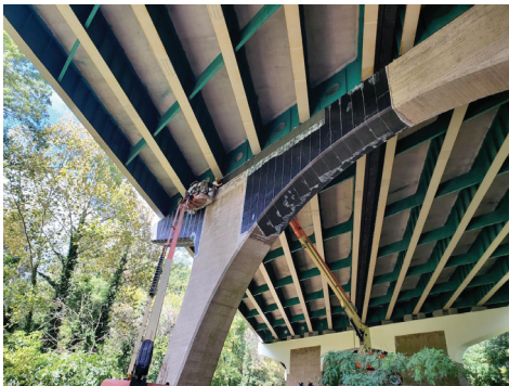
Installation of Fyfe’s Tyfo SCH-41 2X CFRP System Above Arch Vertical for Negative Flexural Reinforcement
