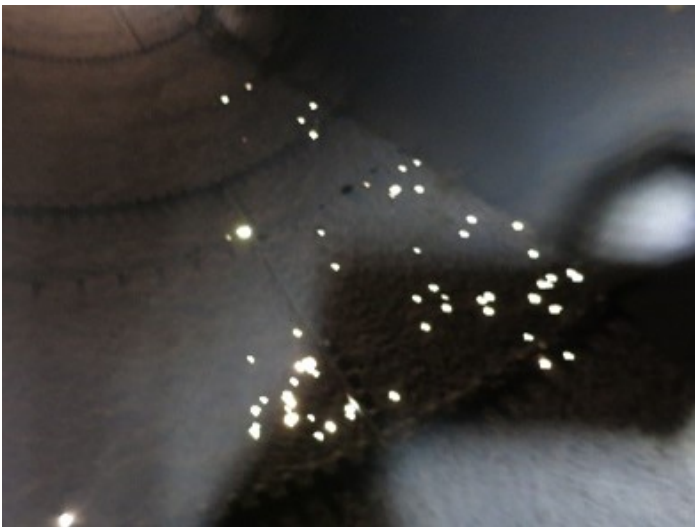
Eagle River Station penstock before rehabilitation showing holes
