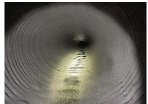
Chula Vista storm drain after rehabilitation. Spincast layer of GeoSpray geopolymer to create a new pipe-within-a-pipe.
