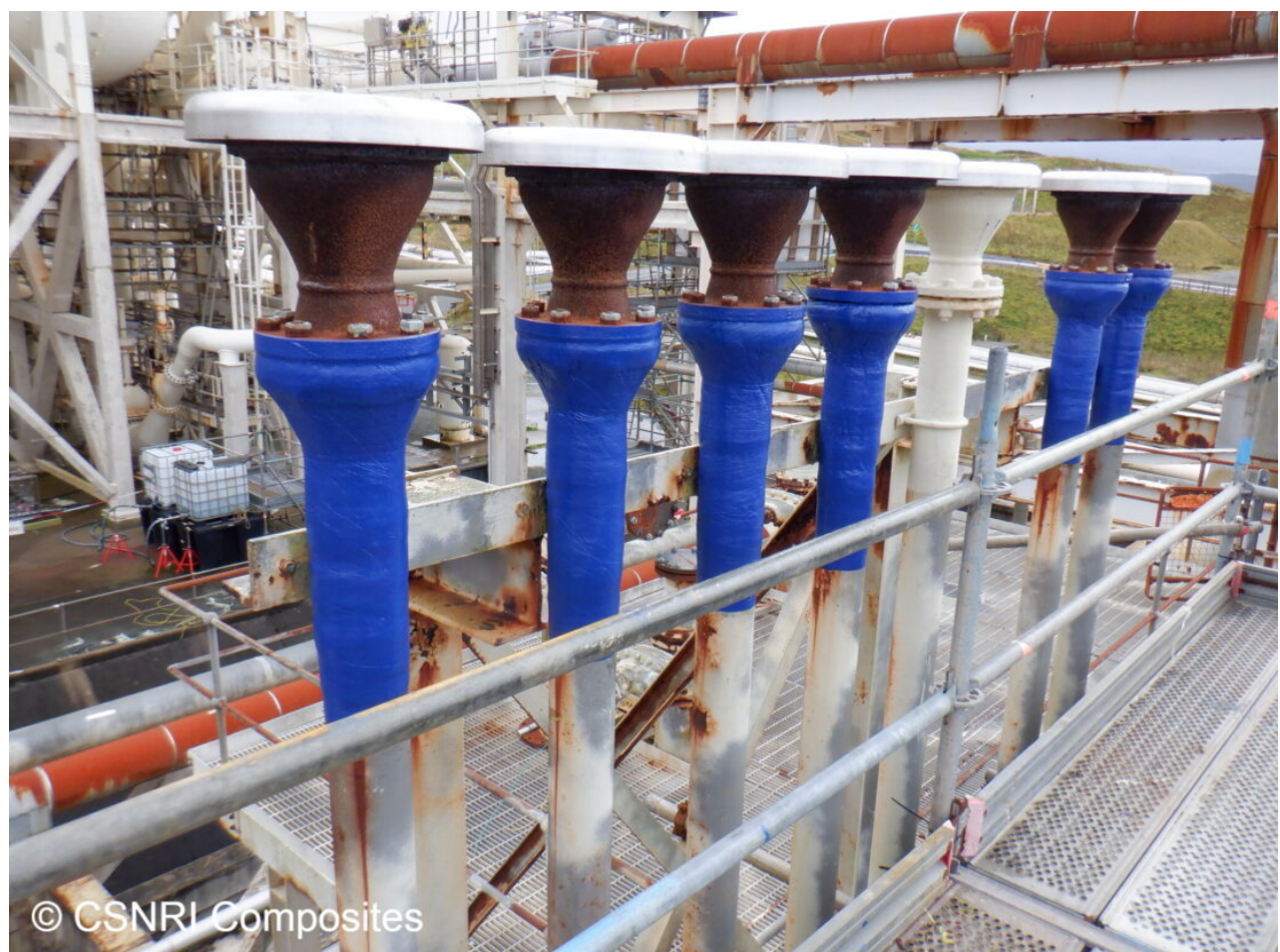
The final repair received an epoxy UV coating for additional protection from harsh weather conditions that are typical of the northern UK area.
