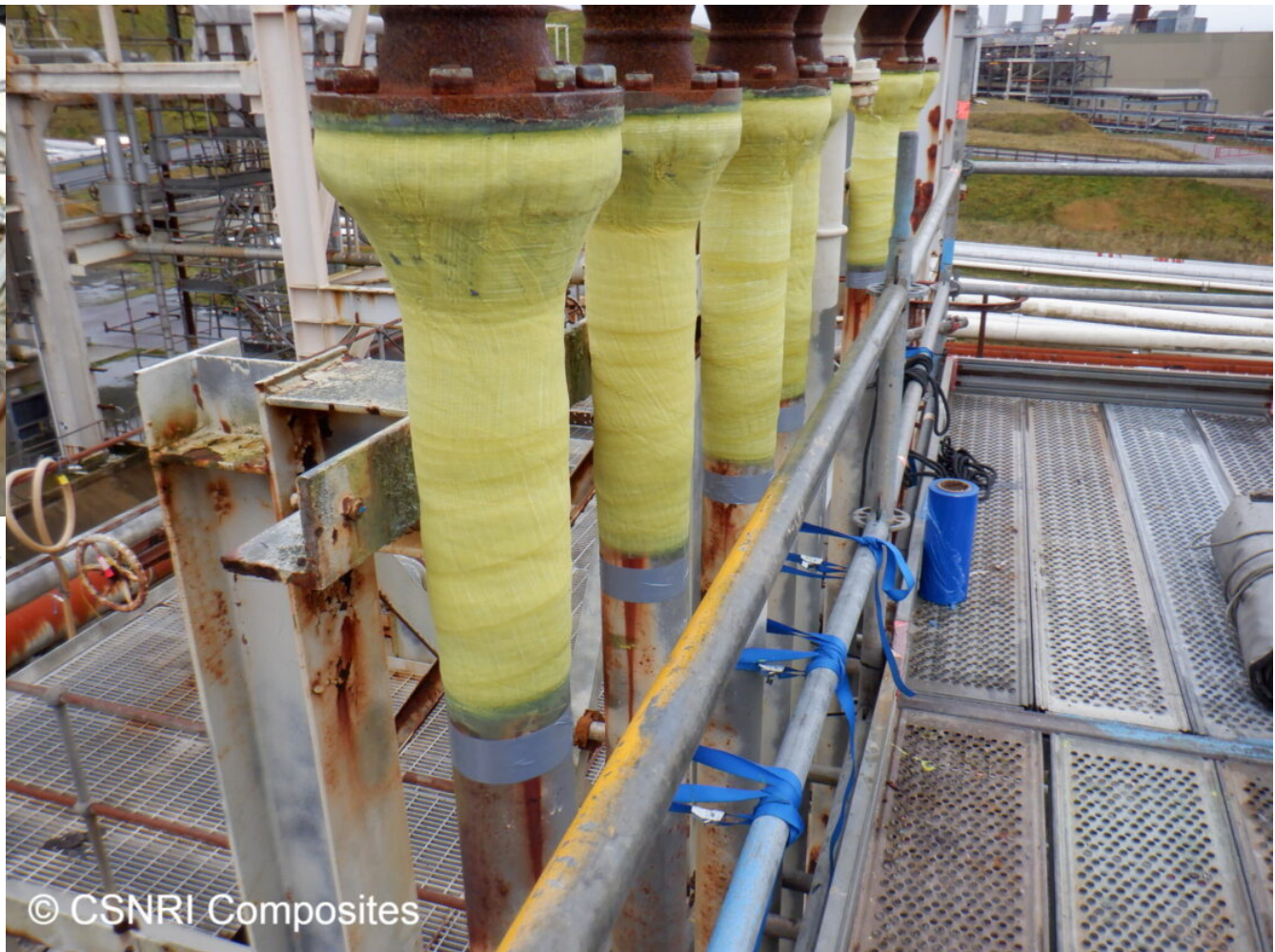
ThermoWrap MT® was field-saturated with six layers applied to each vent stack.
