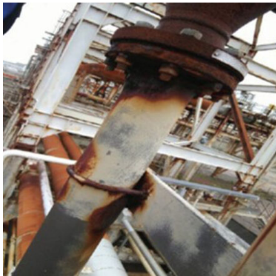
Using a cold-cut method, U-bolts were mechanically cut to improve accesses to areas of corrosion for application of ThermoWrap MT repair.
