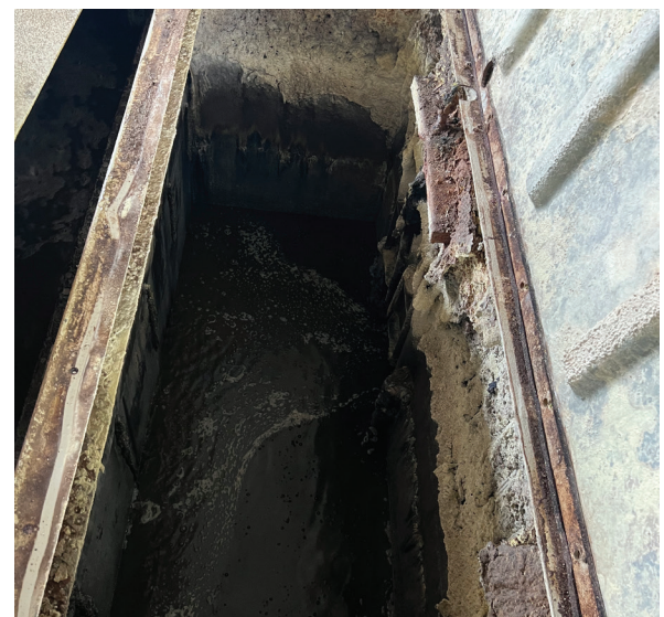
Heavily corroded treatment tank
