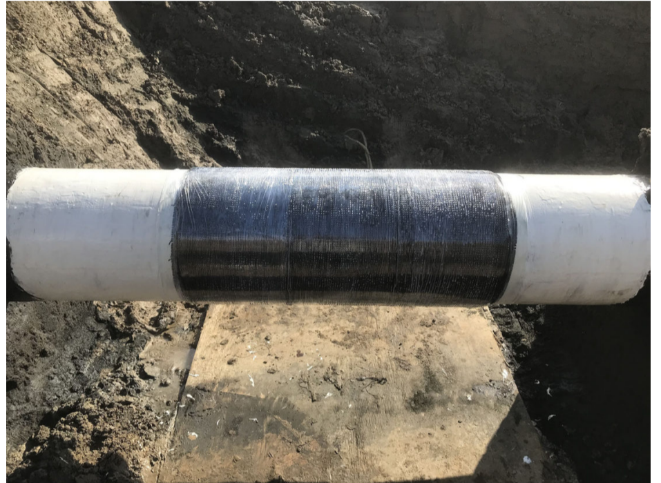
The team installed 24 layers of composite cloth over a 3-ft (1-m) section of pipeline, then covered the repair area with constrictor wrap and perforated it to allow the composite to cure.
