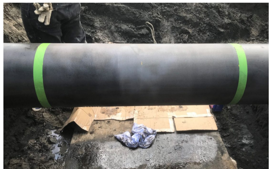
Technicians prepared the pipe surface to a near-white profile and wiped it with acetone in preparation for the composite installation.
