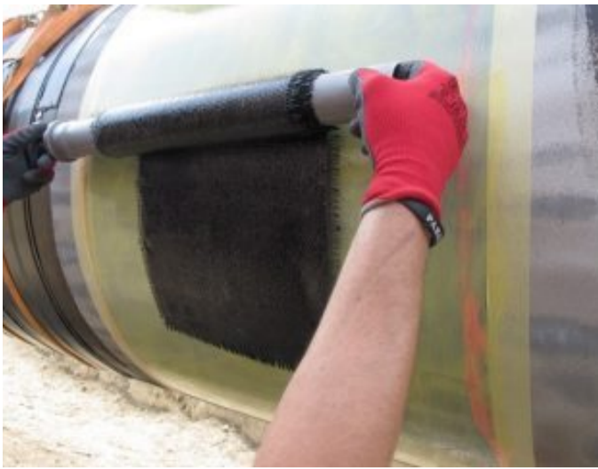
A Clock Spring trained and certified repair technician from SEPS applies DiamondWrap® to the damaged pipe.
