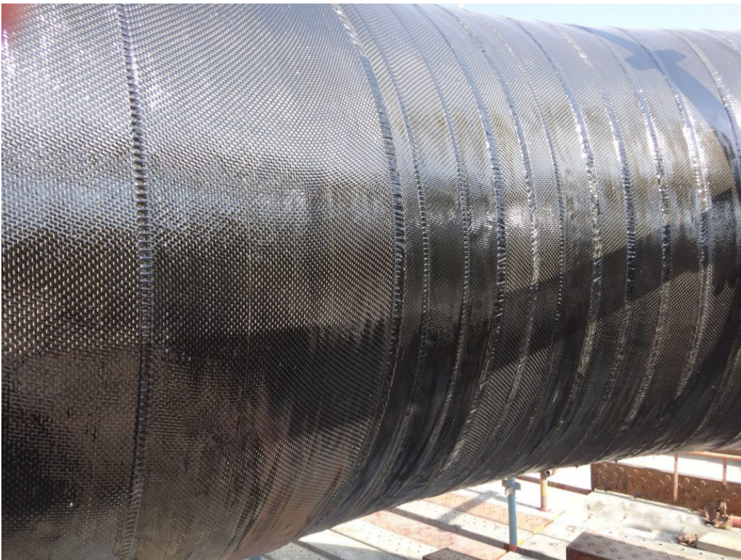
A closeup of the repaired line shows how the carbon fiber was wrapped around the line. The repair team covered the surface of the damaged area with two layers of carbon fiber affixed with HTA epoxy. (Photo courtesy of ClockSpring|NRI)
