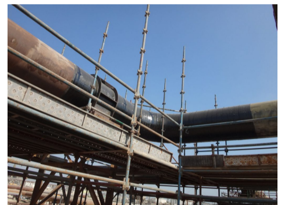
A team of 24 trained and certified installers worked from scaffolding erected around the elevated line to execute the repair. (Photo courtesy of ClockSpring|NRI)
