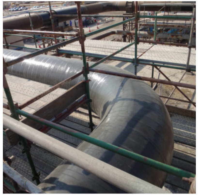
Despite being installed in a very hot environment where temperatures exceeded 45° C (113° F), the composite system cured perfectly, restoring the line to safe operations without introducing hot work and with no negative environmental consequences. (Photo courtesy of ClockSpring|NRI)
