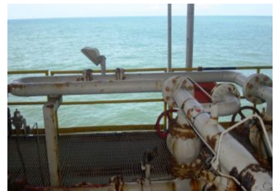
The Prover Loop comprises five spool pieces, where corrosion had created multiple pinhole leaks.
