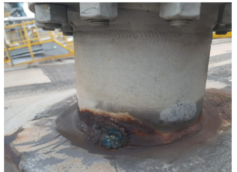
Girth Weld Damage
