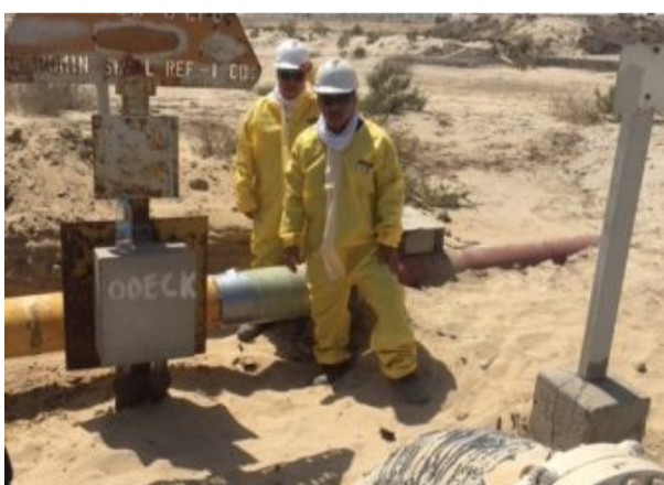
A team of Clock Spring trained and certified installers applied the Contour repair.
