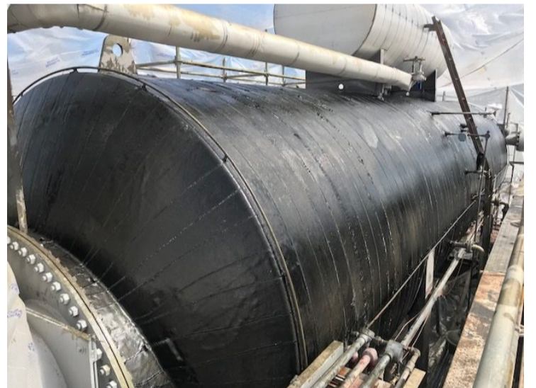
The flexibility and low profile of the DiamondWrap composite system allow installation even in areas with limited clearance. (Photo courtesy of ClockSpring|NRI)
