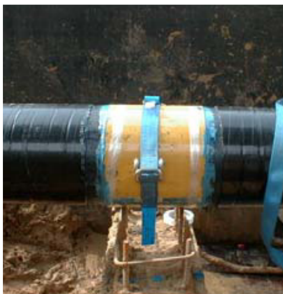
Three layers of Clock Spring at each support location of newly laid pipe prevented corrosion from concrete
