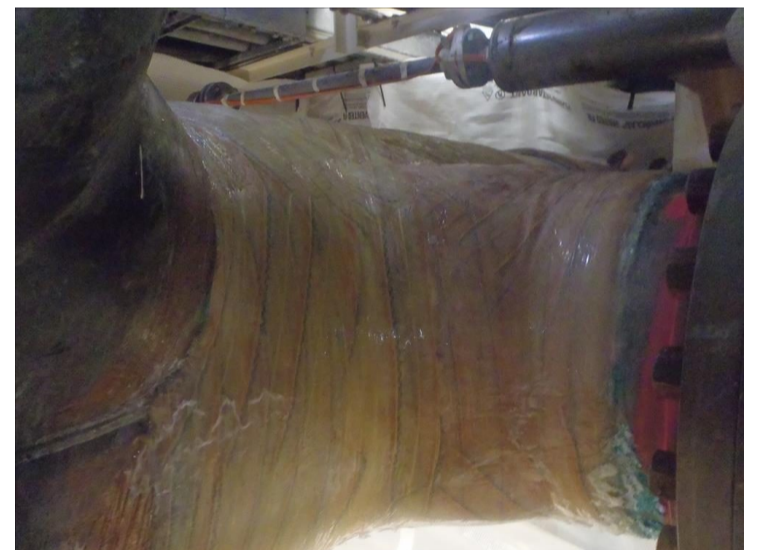
The repair executed by the original solution provider failed to arrest the leaks in the high-pressure line.
