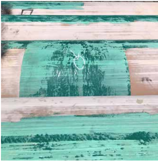
Figure 1. Pipeline with only epoxy coating was pulled twice, resulting in damage to the steel in both cases. When Scar-Guard was applied to the line for the third attempt, the installation was carried out without incident. Photo courtesy of CSNRI.
