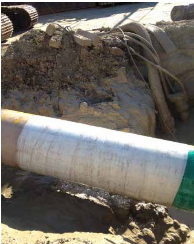
Figure 2. After the line was installed with Scar-Guard applied, it was pulled back and examined for damage. A close inspection revealed that Scar-Guard provided the necessary protection to ensure a successful job.
