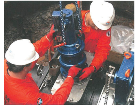
Alterations to the EZ Valve allowed installation on the irregular dimensions of the old cast iron main.
