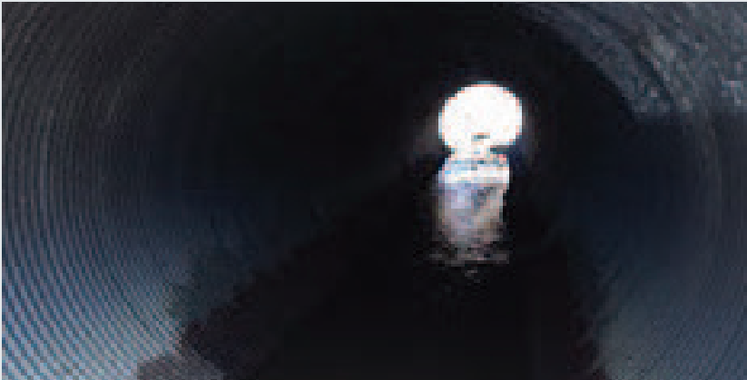
Existing invert with pitting and corrosion.
