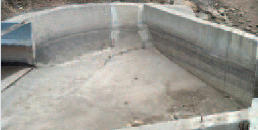
Existing damaged drainage structure prior to lining.
