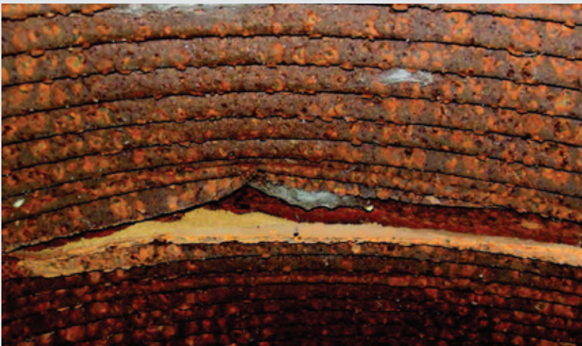
Initial conditions - pipe joint separation.
