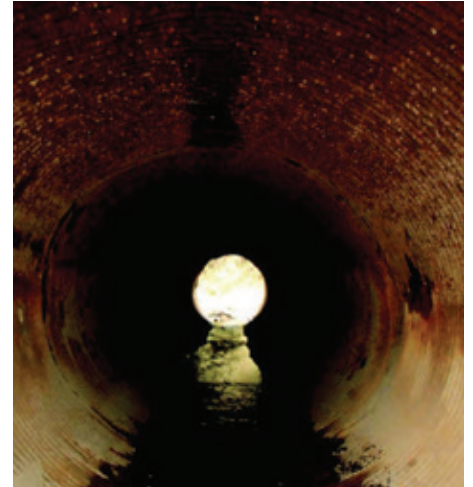
Initial pipe condition with significant invert corrosion.
