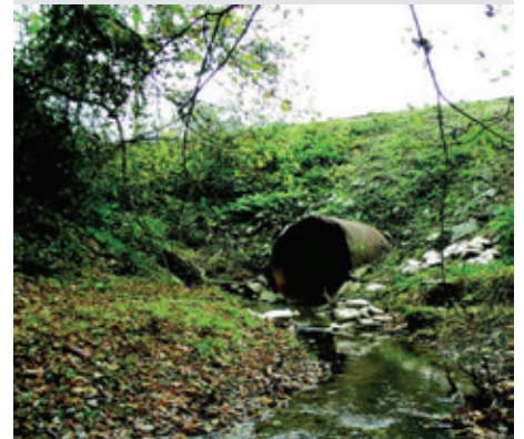
The NCDOT was faced with significant issues of culvert failure and bank erosion.
