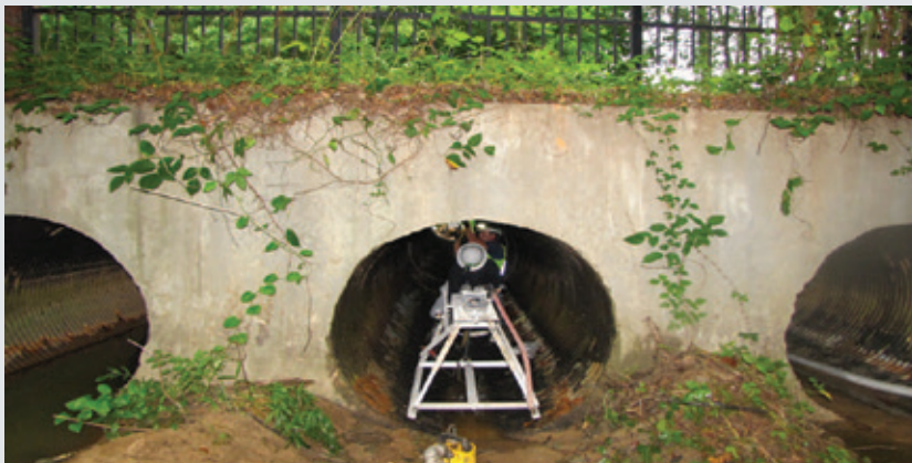
The casting equipment being positioned in the pipe prior to GeoSpray mortar application.
