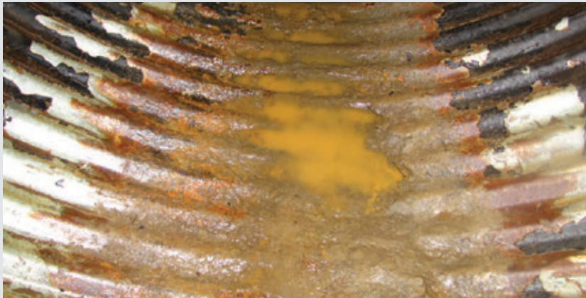
Corrosion of the CMP invert.
