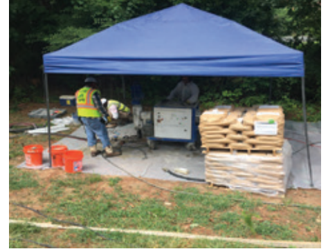
The footprint of the equipment allowed for the roadway to remain open.
