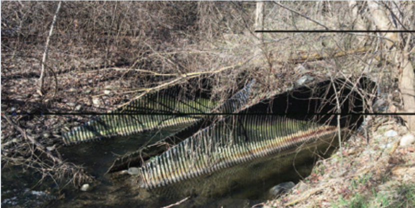
Deteriorating existing culverts.
