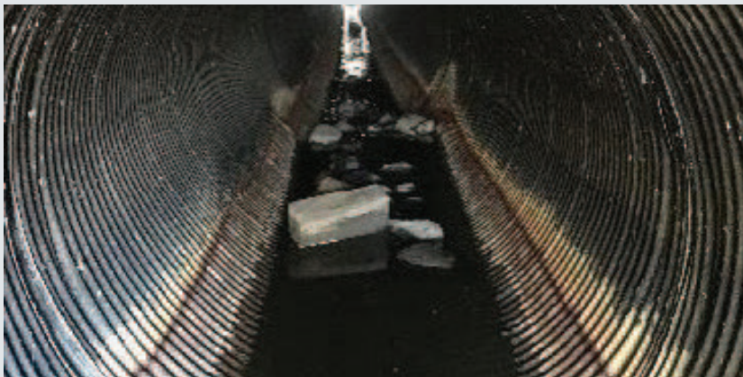
Debris and deterioration within culvert.
