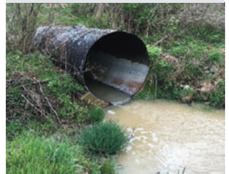
The 78-inch CMP culvert had a cracked and worn invert that showed severe ovality.
