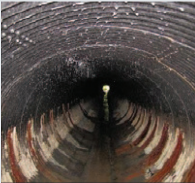
Initial pipe conditions were extremely poor.
