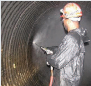
Drips for the asphalt were removed and the loose material was pressure-washed off.
