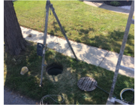
Typical manhole application in right-of-way with tripod set up.
