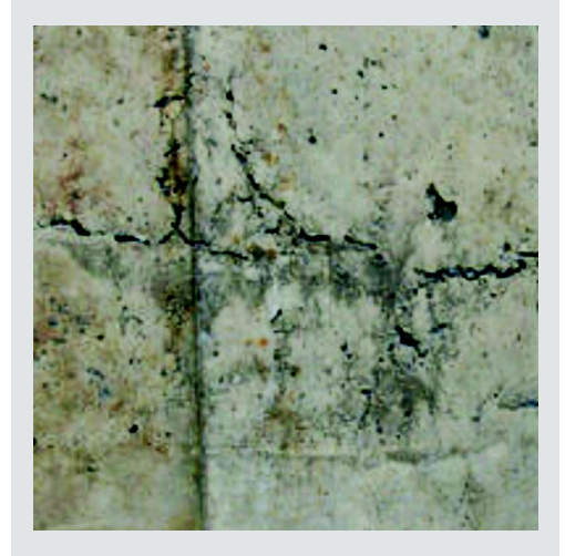
Figure 1. An example of a cold joint formed in a concrete wall.
