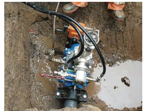
Using the newly installed left close, 4-inch (100-mm) AVT EZ Valve will make future maintenance less intrusive, less complicated, and less expensive.
