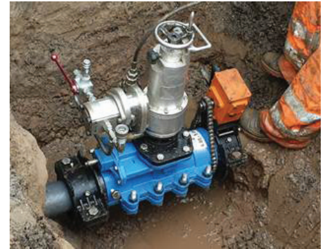
Three technicians installed the 4-inch (100-mm) AVT EZ Valve on a PVC clean water main in 3 hours, delivering a durable solution without interrupting service.
